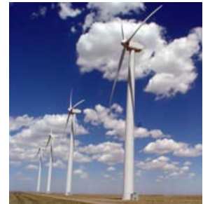
3-Bladed wind turbine-
